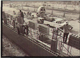
1972 Construction begins on a combination parking structure and athletic field in Pasadena.
